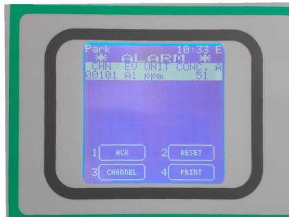
Figure 21) Typical ALARM state of the ACTIVE EVENTS screen.
