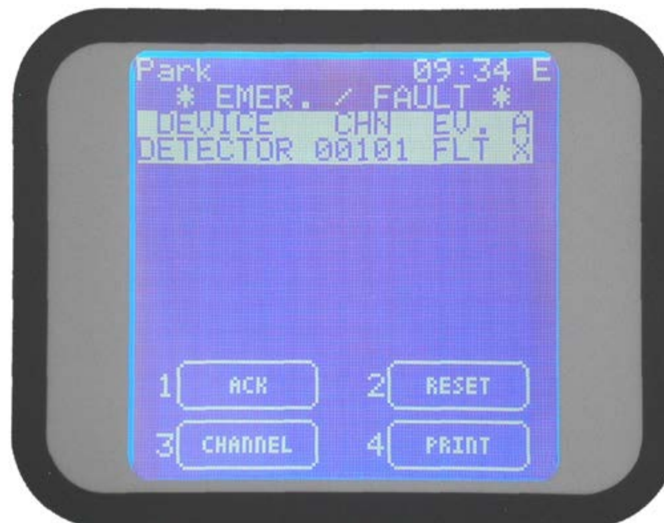
Figure 23 Typical FAULT state of the ACTIVE EVENTS screen.
