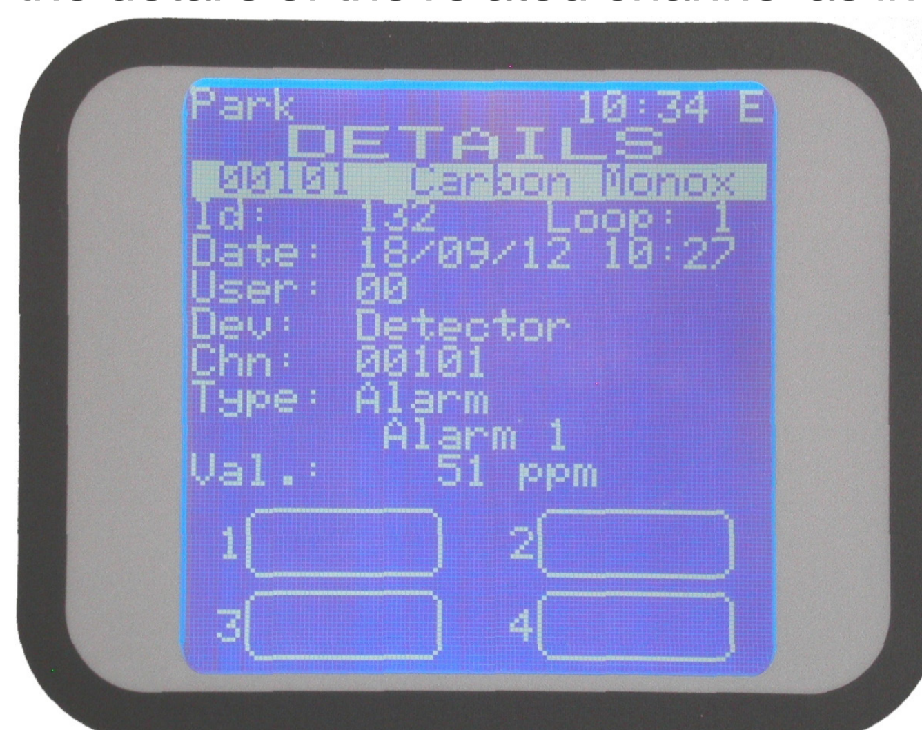
Figure 24 ALARM details screen.
