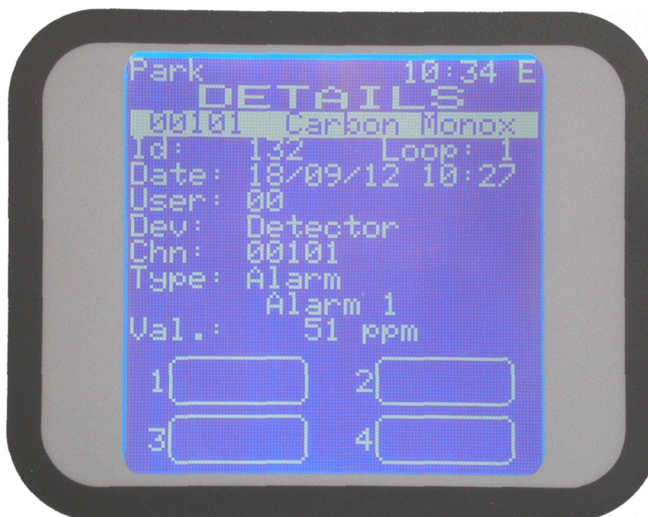
Figure 26 FAULT details screen
