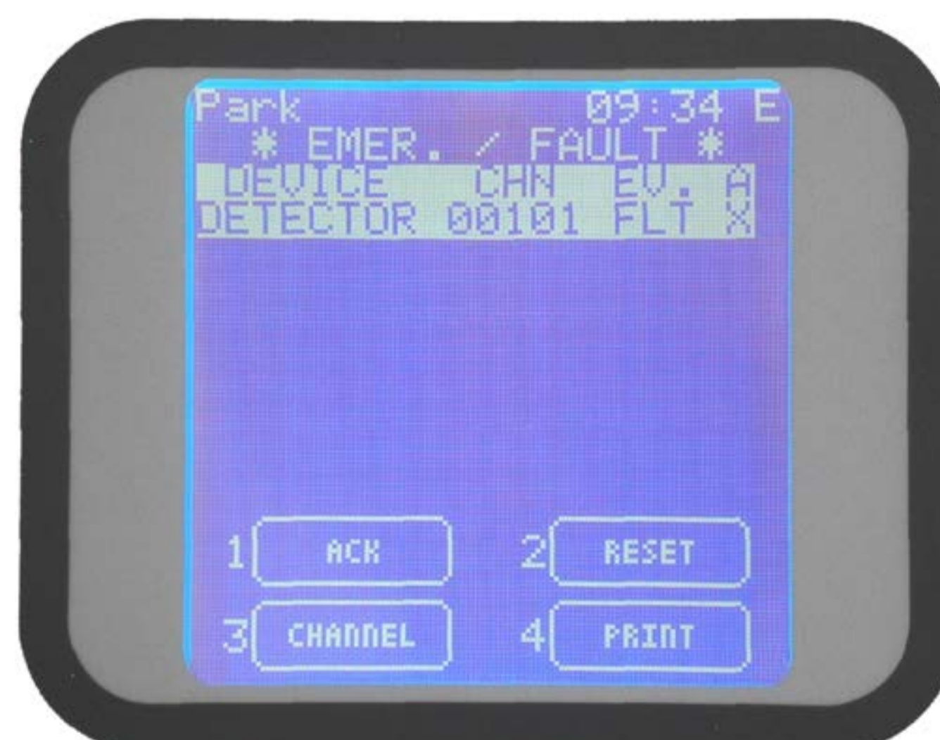
Figure 24 Typical FAULT state of the ACTIVE EVENTS screen.
